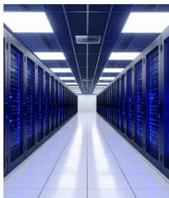
Data centres & critical infrastructure
